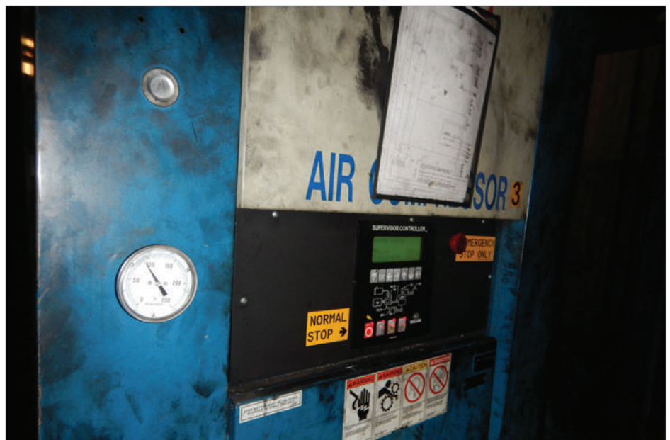
Figure 6: To better control this compressor of another brand, IAC integrated a Sullair microprocessor and Airleader took direct control of the poppet valves to control part loading of this unit.
