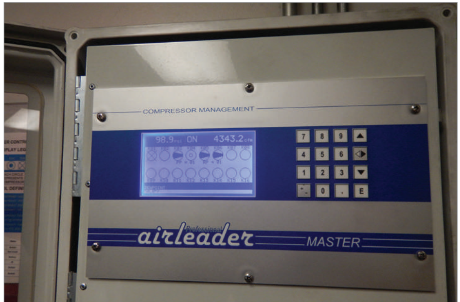
Figure 5: This controller runs the air compressors with best efficiency at full load and varies the flow of the compressors with variable capacity control.
